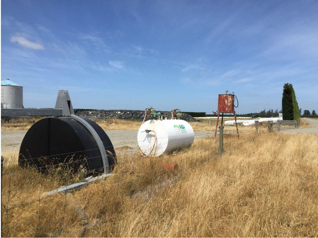
Photograph 3: (Fuel storage tanks, historical (red tank) and current (white))
